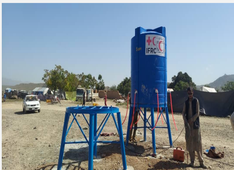
With the support of IFRC, ARCS installed 20 water tanks in 10 villages of Barmal district of Paktika province (Photo: ARCS)
