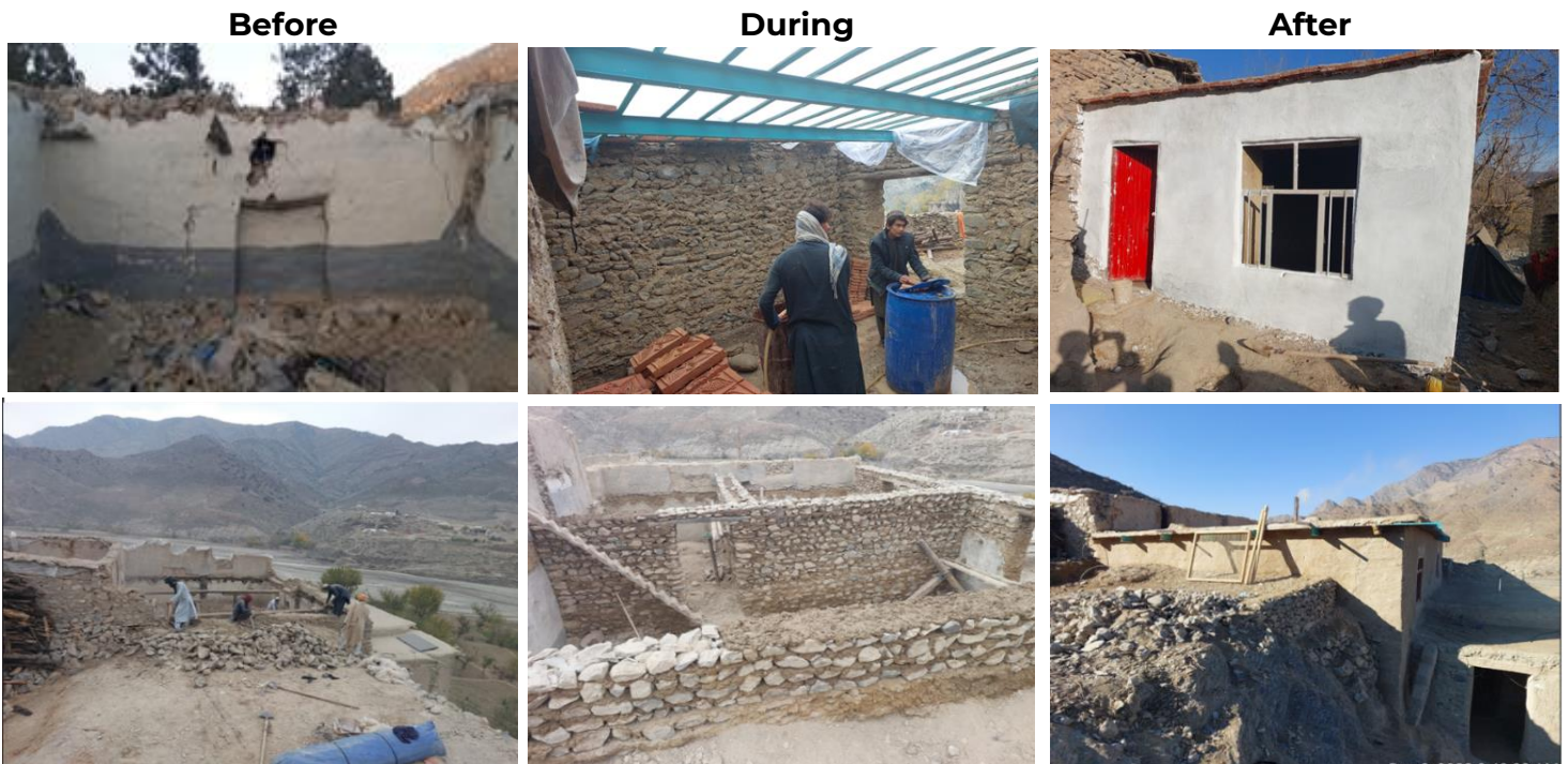
More than 2,000 households repaired their houses with the financial and technical support from ARCS/IFRC in Khost and Paktika provinces of Afghanistan in 2022. The shelter repair was completed before onset of the harsh winter in the affected areas. (Photo: IFRC)
